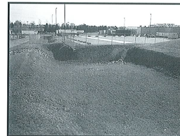
Traditional stormwater basins offer little in the way of aesthetics or ecological value. (Photo: LandStudies, Inc)
